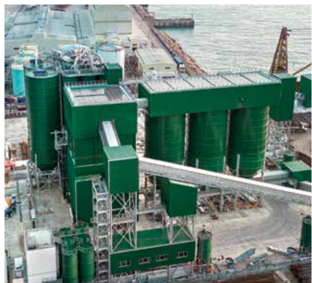
In December 2022, Alliance started full operation of its new Sai Tso Wan 2 mega concrete plant in Hong Kong.
