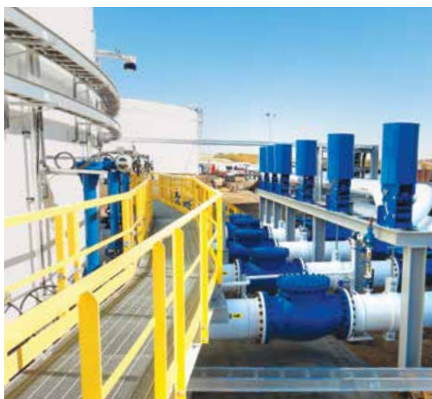
Canadian Midstream Assets completed the construction of the Onion Lake lateral in March 2022.
