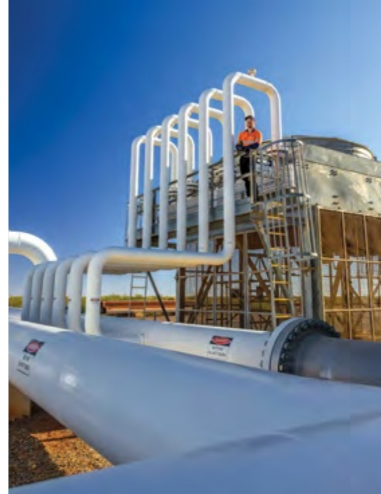
Australian Gas Networks is one of Australia's largest natural gas distribution companies. It owns over 27,000 kilometres of distribution networks and 1,000 kilometres of transmission pipelines.
