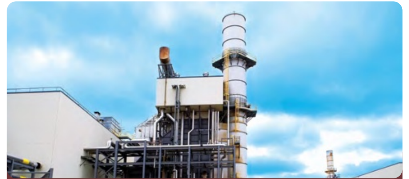
Canadian Power’s Meridian Cogeneration Plant operated smoothly under the power purchase agreement for the provision of electricity to SaskPower and thermal energy to Cenovus.
