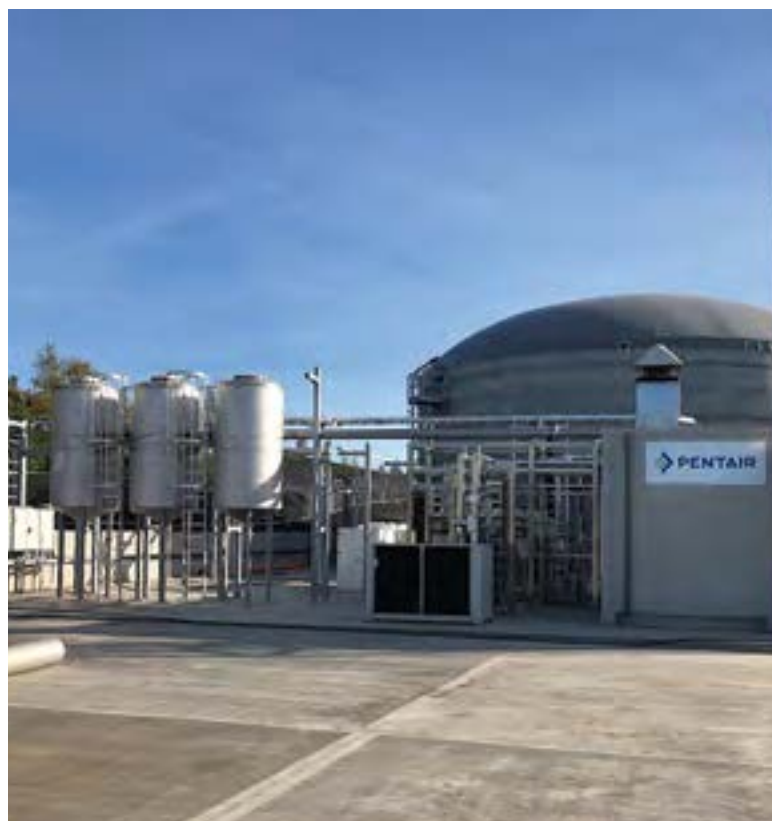
Northern Gas Networks' HyDeploy project has commenced blending hydrogen with natural gas on a public gas network.
