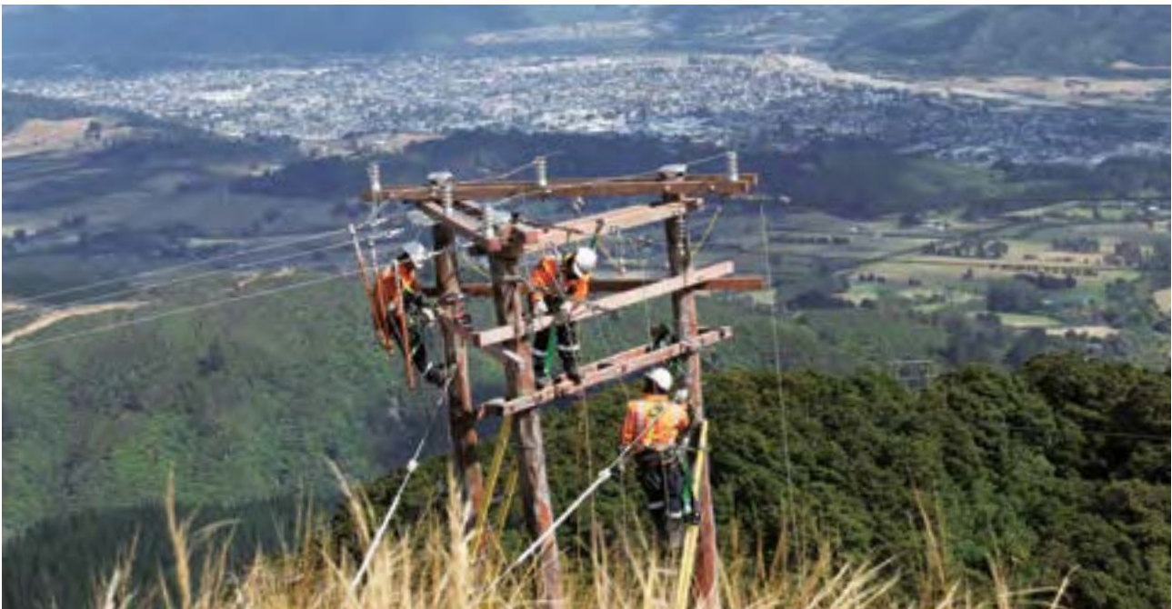
Wellington Electricity's three-year Earthquake Readiness Programme was completed in the first quarter of 2021.
