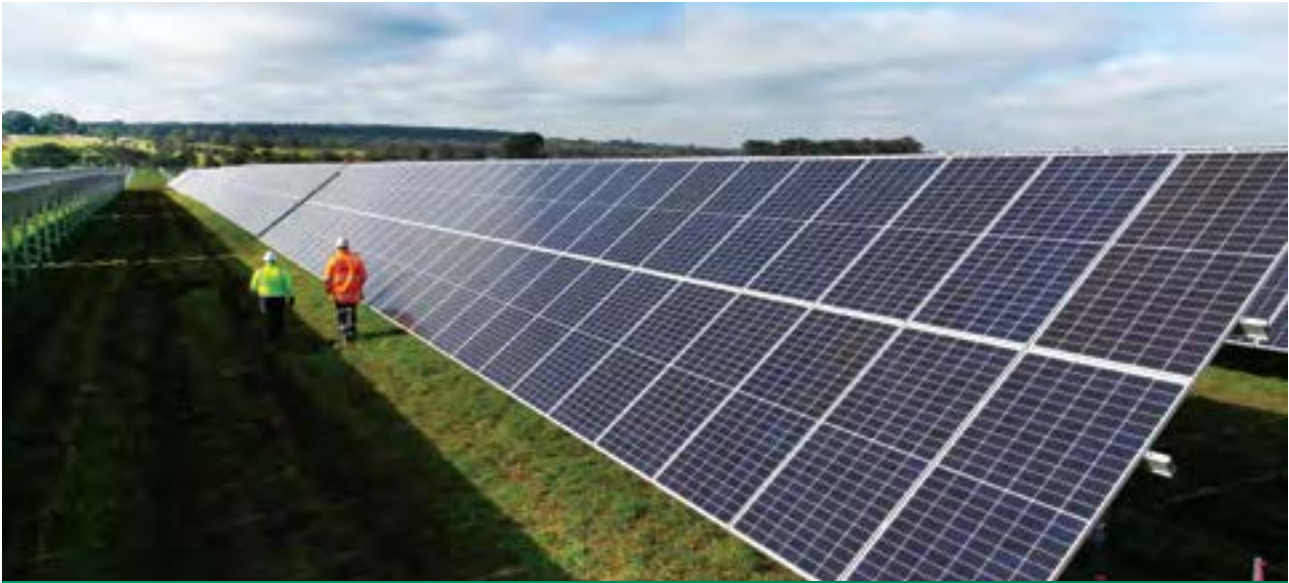
Victoria Power Networks' Beon completed the construction of the 62 MW Jemalong Solar Farm, 106 MW Yatpool Solar Farm and the 12 MW Melbourne Airport Solar Farm, the latter being one of the largest behind-the-meter solar installations in Australia.
