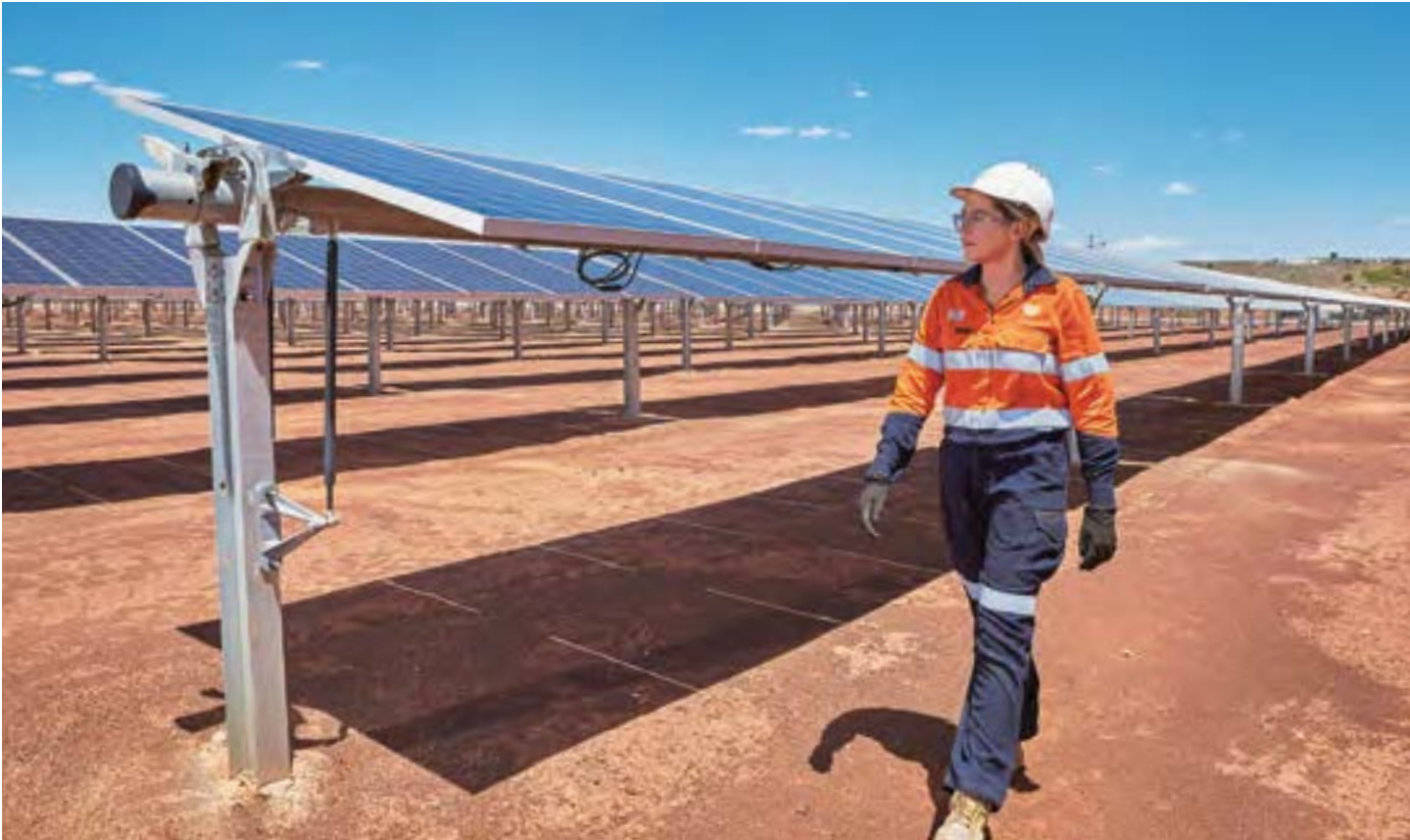
The Northern Territory Government commissioned EDL to construct, own and operate a new hybrid renewable power station which includes solar power and battery to provide the town of Jabiru with reliable energy.
